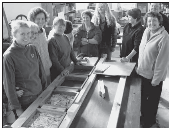
Building the concrete formwork for the mosaic tiles are, left to right: Kim Mullen, Marg Rehorn, Lesley Anderson, Maery Gabriel, Ingrid Thomas, Anne Napier, Yvonne Maygar, Christina Rasmussen and Marree Wallace.
